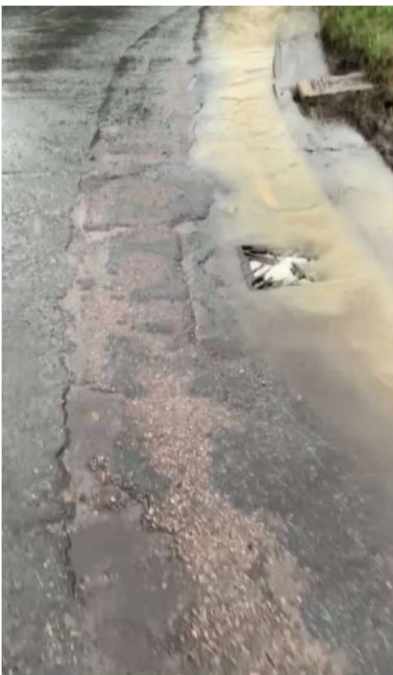
- gulley blocked / not working
